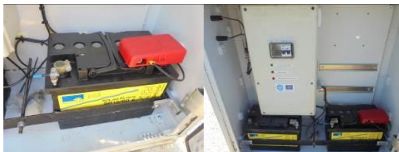
Figure 20. Corrosion effect in batteries connection
