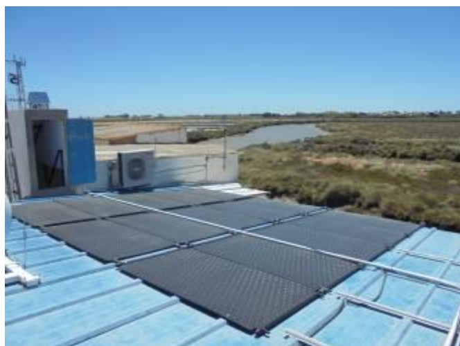
Figure 22. AQUASEF solar thermal installation
