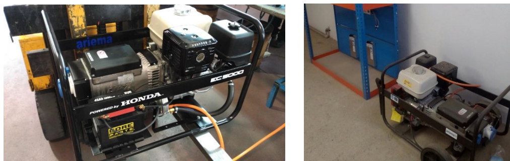
Figure 29. ICE Power generator during transformation works and in AQUASEF facility The chosen engine is a very accessible Honda model (GX390). Preliminary works took place throughout 2015 and early 2016 (left), and then installation and field-testing (right).
