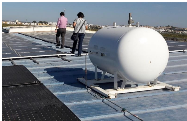
Figure 27. Hydrogen pressurized tank
